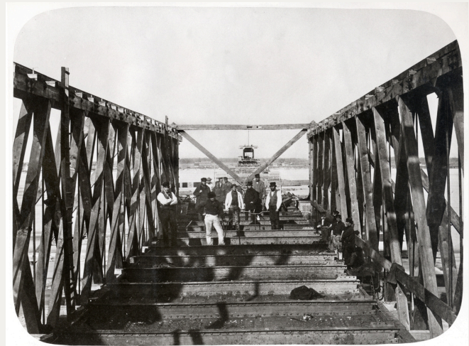
William Notman (1859). Framework of tube and staging no. 8, Victoria Bridge, Montreal, QC, 1859 , https://collections.museum-mccord-stewart.ca/en/objects/106938/structure-du-tube-et-echafaudage-no-8-pont-victoria-montre?ctx=4b5a9753f184a4c06dbd2425326bc8214a6f0bb0&idx=55
